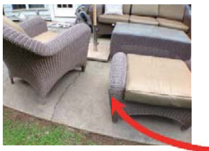
Rear Exterior Patio/Porch Crack up the middle.
