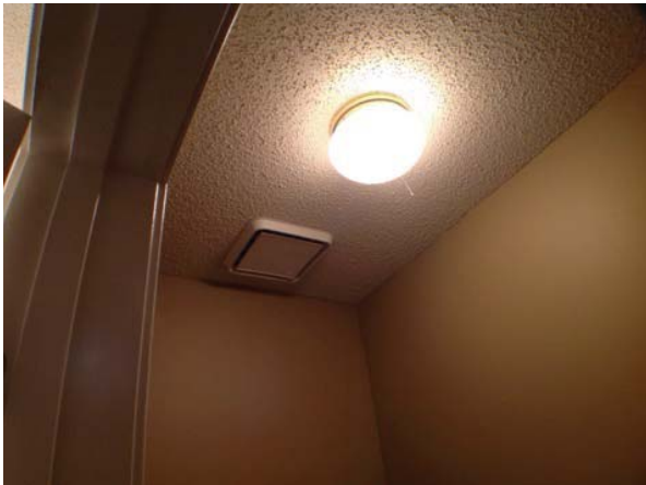
Exhaust Fan - In commode room.
