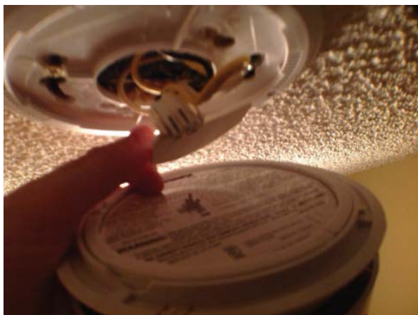
Smoke Alarm - Wrong connection, but still functions.
