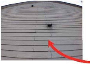
Front Exterior Walls/Siding/Trim Caulked joints of siding are cracking.
