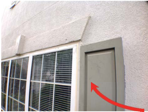
Walls/Siding/Trim - Discolored trim and caulk.
