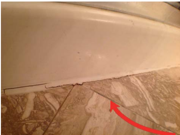
Shower/Fixture - Cracking Caulk on exterior of shower tray.
