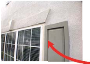
Front Exterior Walls/Siding/Trim Discolored trim and caulk.
