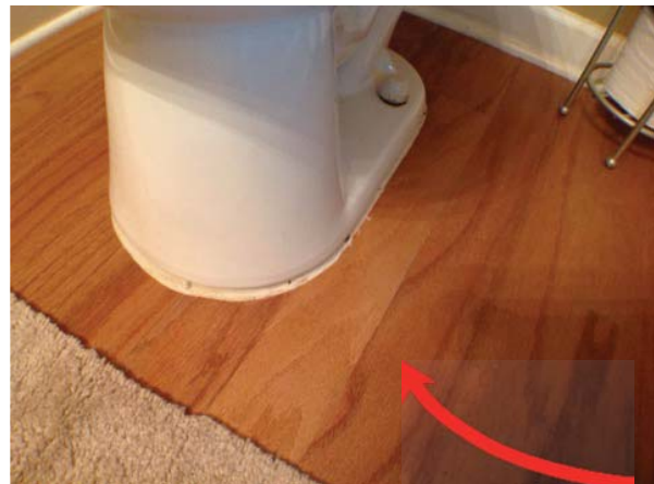
Commode - Discolored and cracking caulk.
