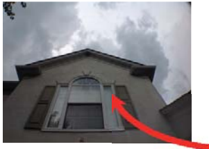
Front Exterior Walls/Siding/Trim Cracking trim above window.
