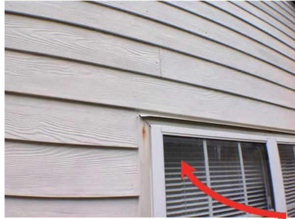
Walls/Siding/Trim - Rear window trim is cracking and discolored.
