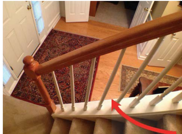
Banister - Banister is loose.
