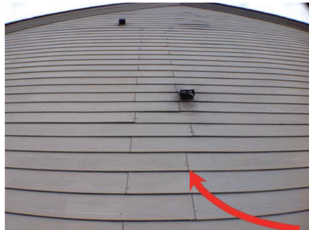
Walls/Siding/Trim - Caulked joints of siding are cracking.
