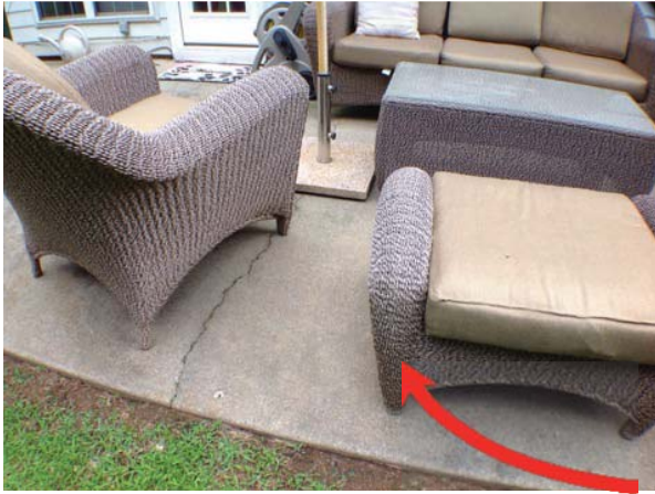
Patio/Porch - Crack up the middle.
