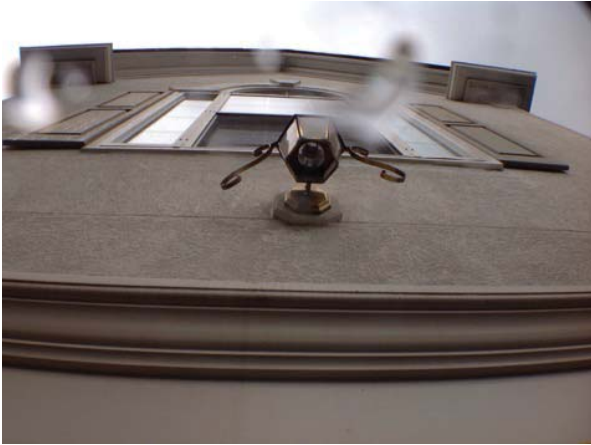
Light Fixtures - Does not turn on.
