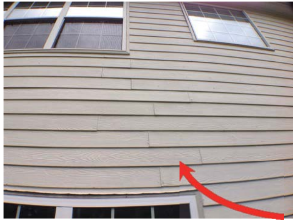
Walls/Siding/Trim - Caulked joints of siding are cracking.
