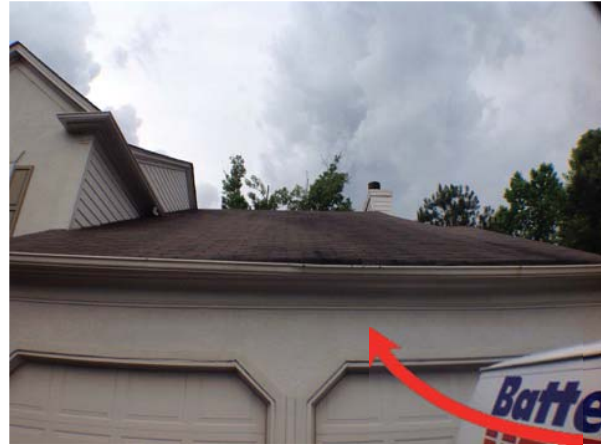
Roof/Trim - Bent Gutter
