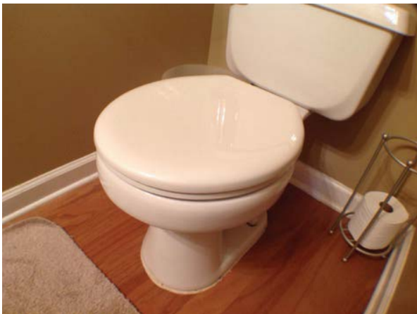
Commode - Caulk at floor is discolored.
