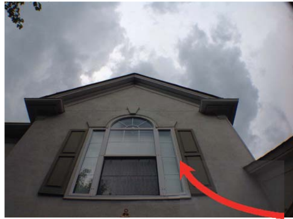
Walls/Siding/Trim - Cracking trim above window.
