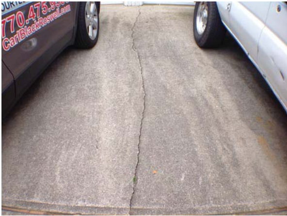
Driveway - Center Crack
