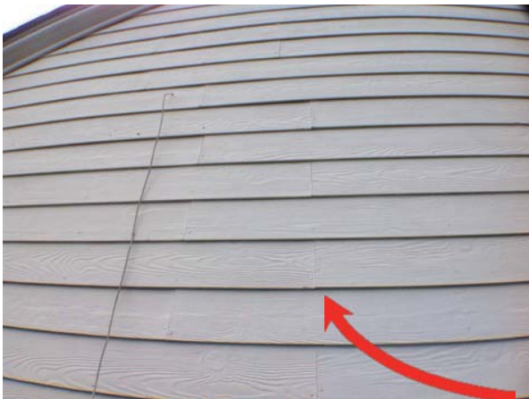
Walls/Siding/Trim - Caulked joints of siding are beginning to crack.
