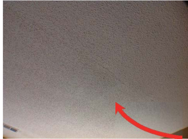
Ceiling - Slight cracking in what looks like an old patch.
