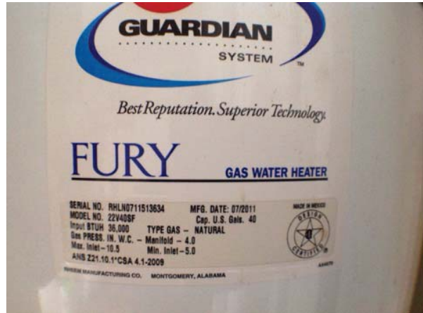
Water Heater - MFG Date
