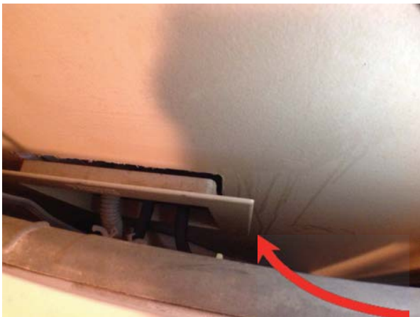
Walls/Paint - Moisture streaks on back wall.
