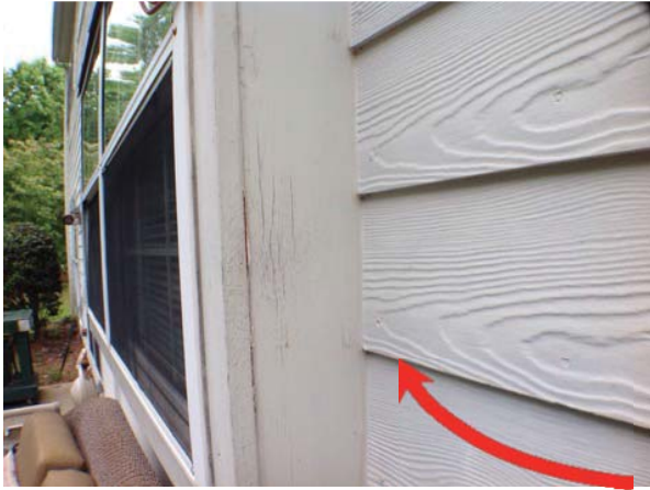
Walls/Siding/Trim - Caulk is separating in rear window bump out.
