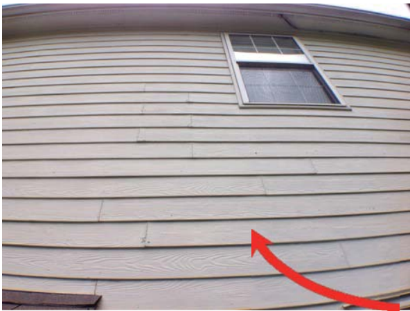
Walls/Siding/Trim - Caulked joints of the siding are cracking.
