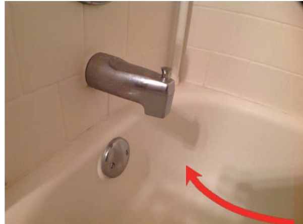
Tub/Fixture - Caulk is slightly Discolored.
