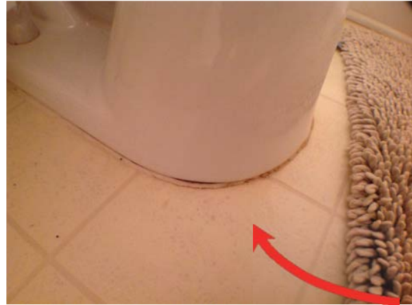
Commode - Discolored caulk and slightly pulling away.
